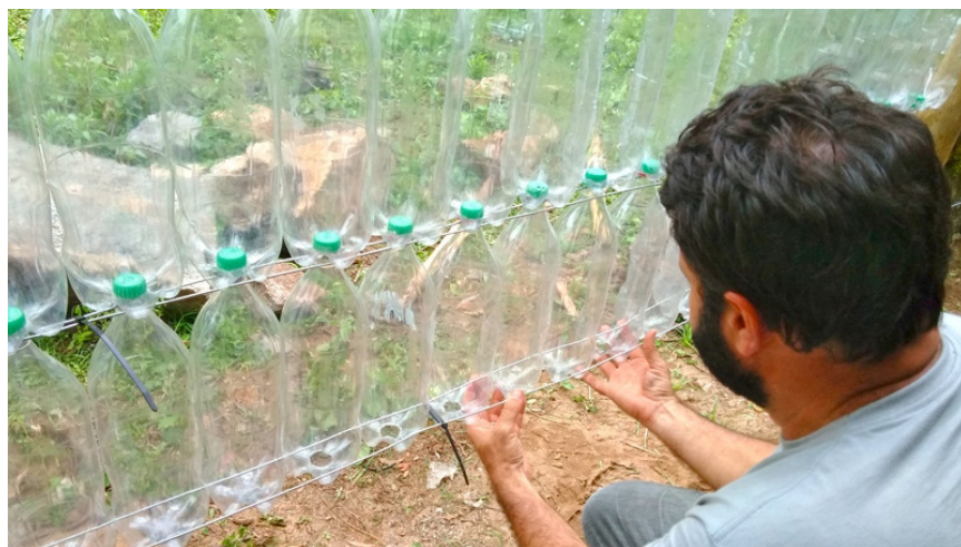
Fig. 11. Construction of the PET Wall in the Botanical Park (courtesy of Ecomuseu Ilha Grande Collection).
