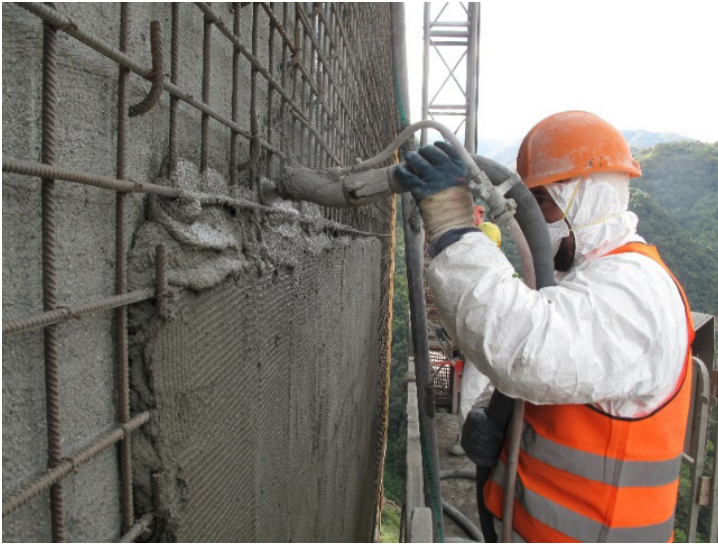
FIG. 20.6 - SPRAY APPLICATION OF MAPEGROUT EASY FLOW ZERO, BY PLASTERING MACHINE EQUIPPED WITH PREMIXER
